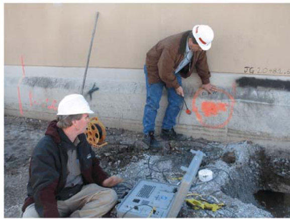
Photo 4 (Fig. 2) - Horizontal impact to side of concrete wall at el. 5 about 0.5 ft below chamfer
