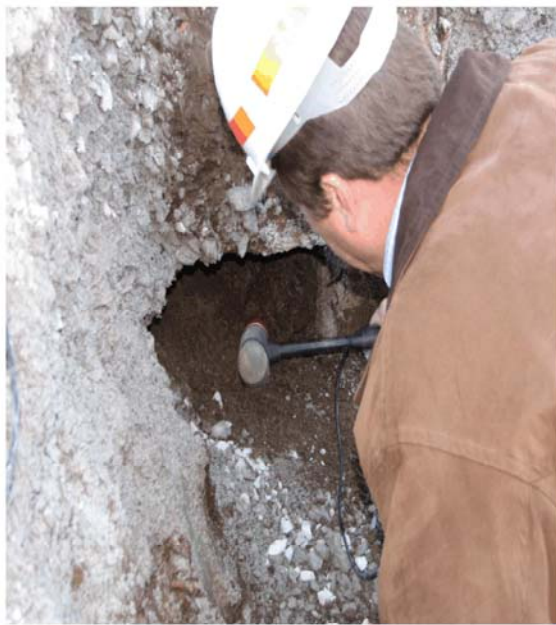
Photo 3 (Fig. 1) - Horizontal impact to sheet pile at 0.5 ft below concrete wall - protected levee side
